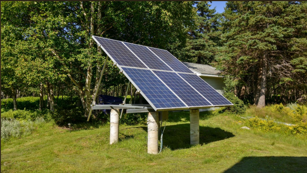
The solar array — off-grid power
